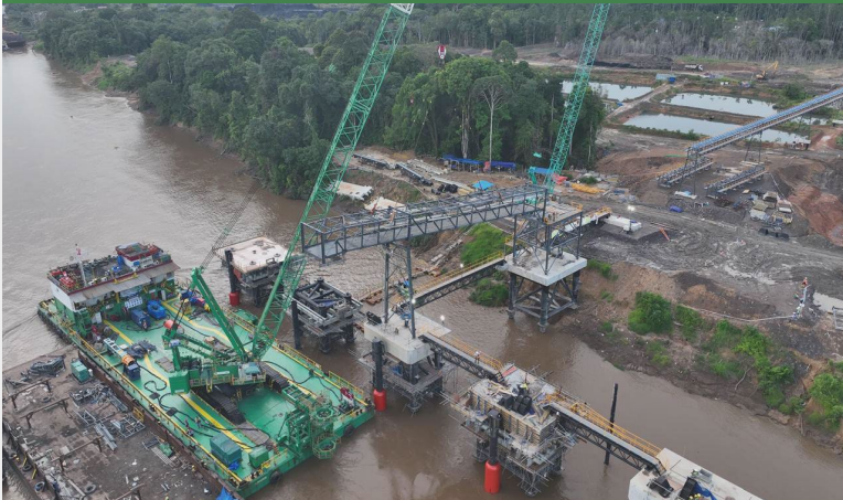
Second Barge Loading Conveyor
