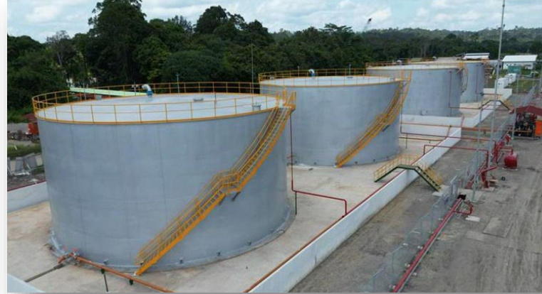
Fuel Storage Tank
